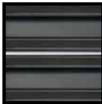
Support beam for cold pool channel
