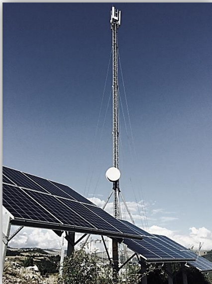
Hybrid Off-Grid Power System EXERON
