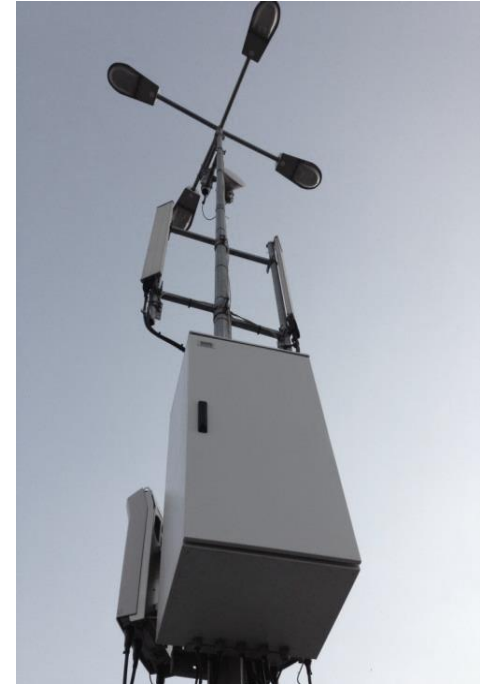
Forced ventilation Single walls
